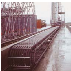
BS3500 chains with supporting frame applied to De Icing equipment at München airport (Germany). The length of the travel distance is 90m and it's velocity is 90m per minute.
